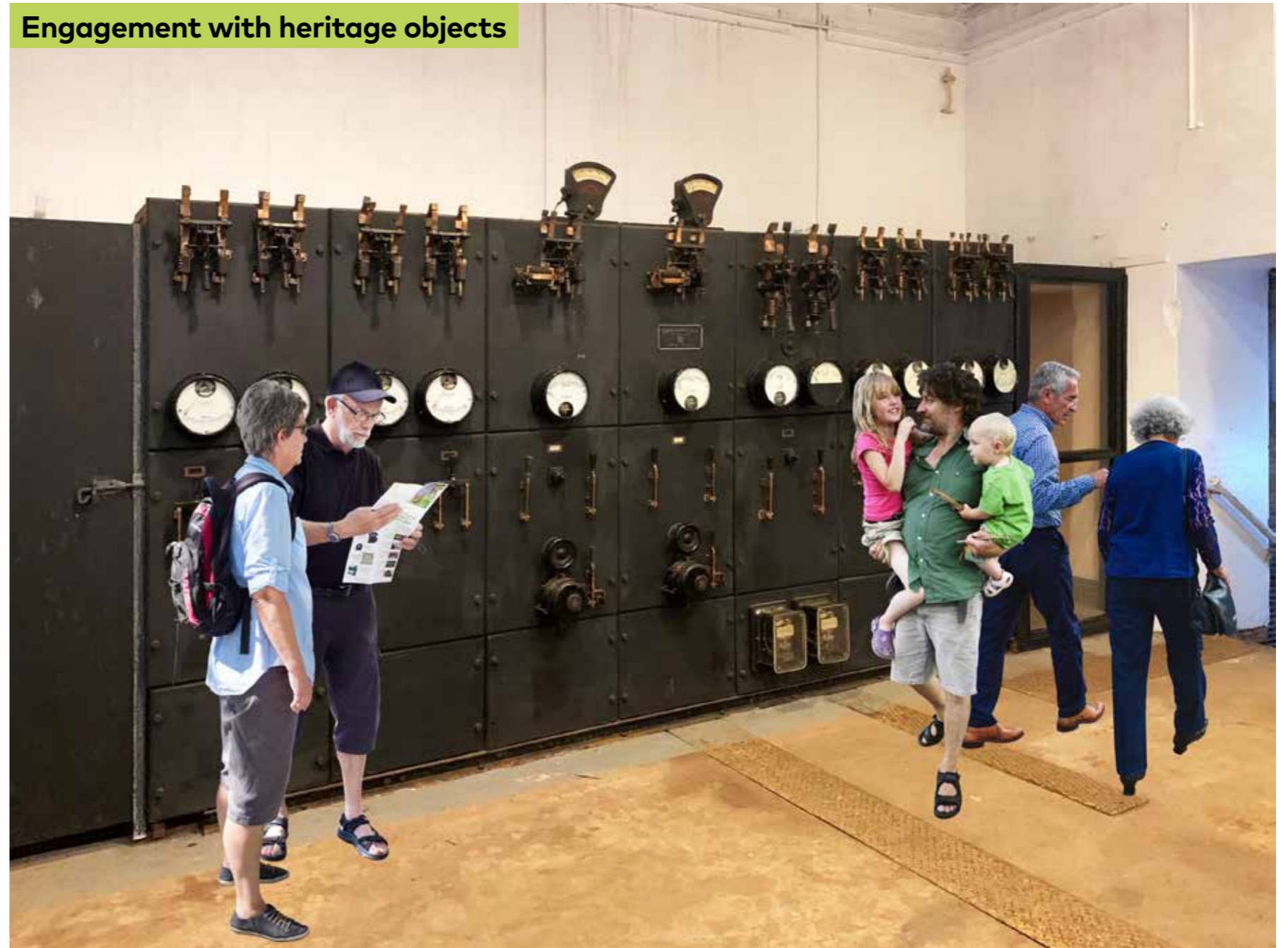
North Fort Engine Room
