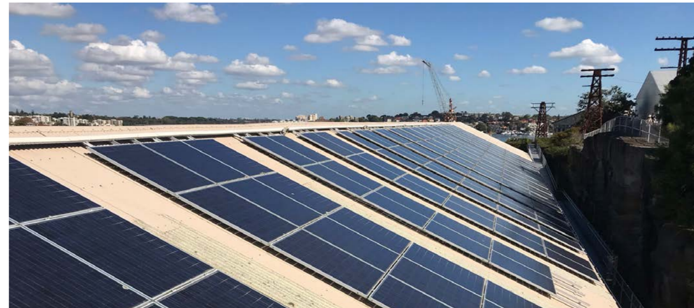
Top and bottom: Solar panels mounted onto the roof of the Turbine Shop at Cockatoo Island / Wareamah. Source: Harbour Trust.
